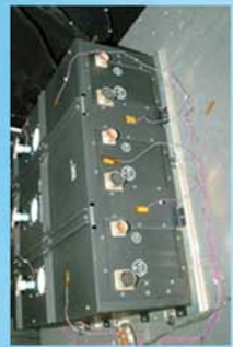
Six batteries Into Bays 2 and 3
